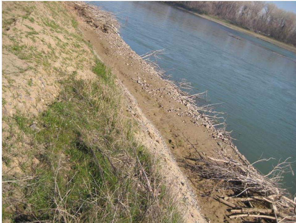
Figure 14. View of top of revetment showing the presence of woody material both on top of the revetment and encased within the structure following the first higher winter flows after construction (Photo taken on 03/12/2008).
