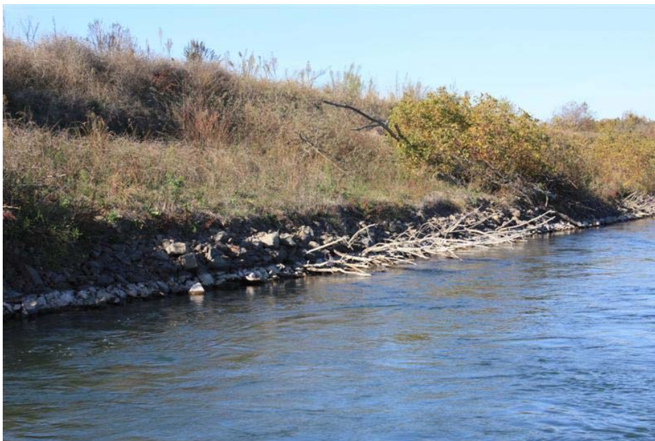
Figure 27. Upstream view of the upper section of the toe rock revetment. Note the large woody debris emplaced on the top of the rock and within the rock during construction and the riparian vegetation that has volunteered onto the top of the rock especially in the vicinity of the large woody debris placed on the top of the rock.
