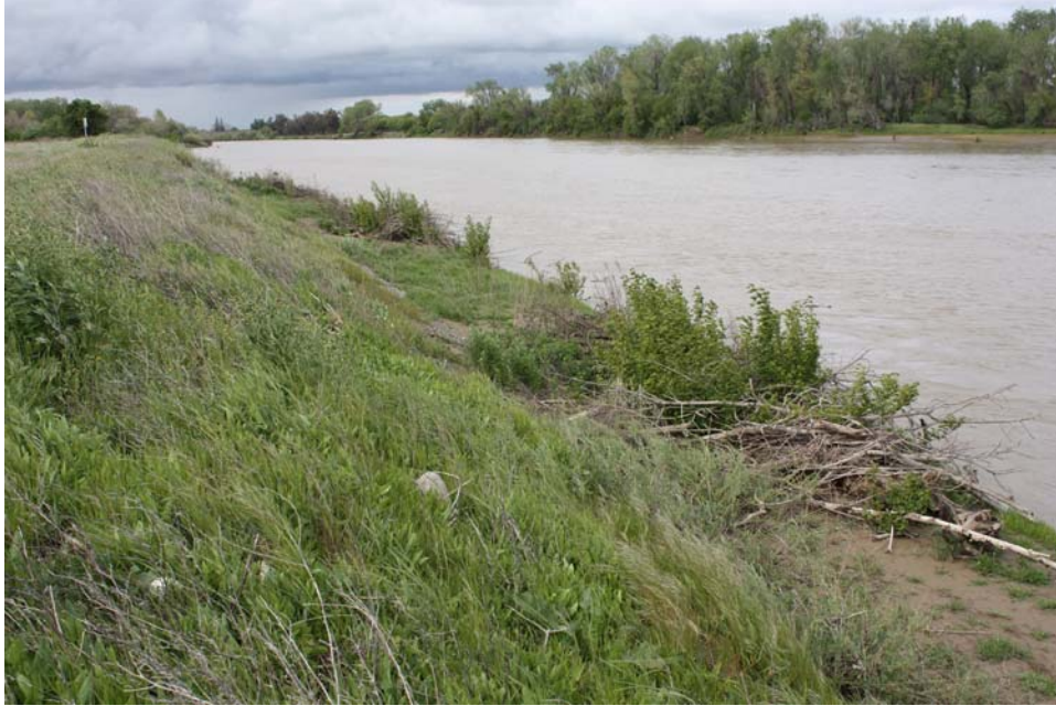
Figure 16. View upstream of the revetment showing the presence of the woody debris piles that were constructed on top of the structure. Flow in the river was about 11,000 cfs (Photo taken on 04/12/2010).
