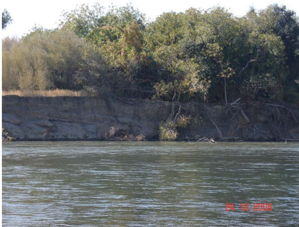
Figure 3. Photograph of the apex of the eroding bend prior to construction of the rock-toe/brush revetment (Photo taken on 10/24/2006).
