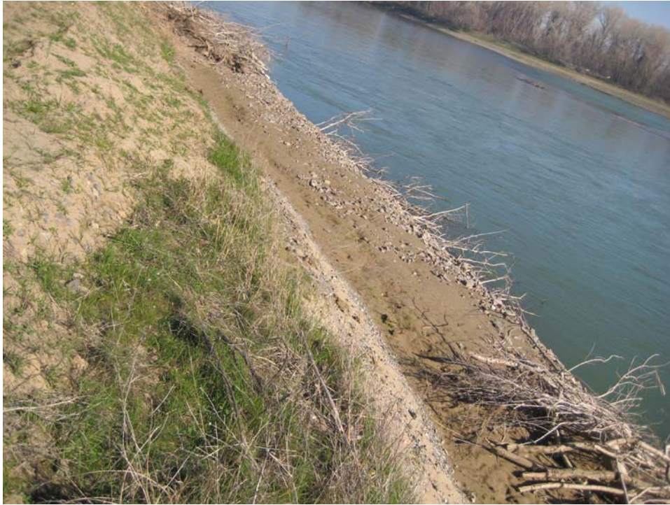
Figure 14. View of top of revetment showing the presence of woody material both on top of the revetment and encased within the structure following the first higher winter flows after construction (Photo taken on 03/12/2008).
