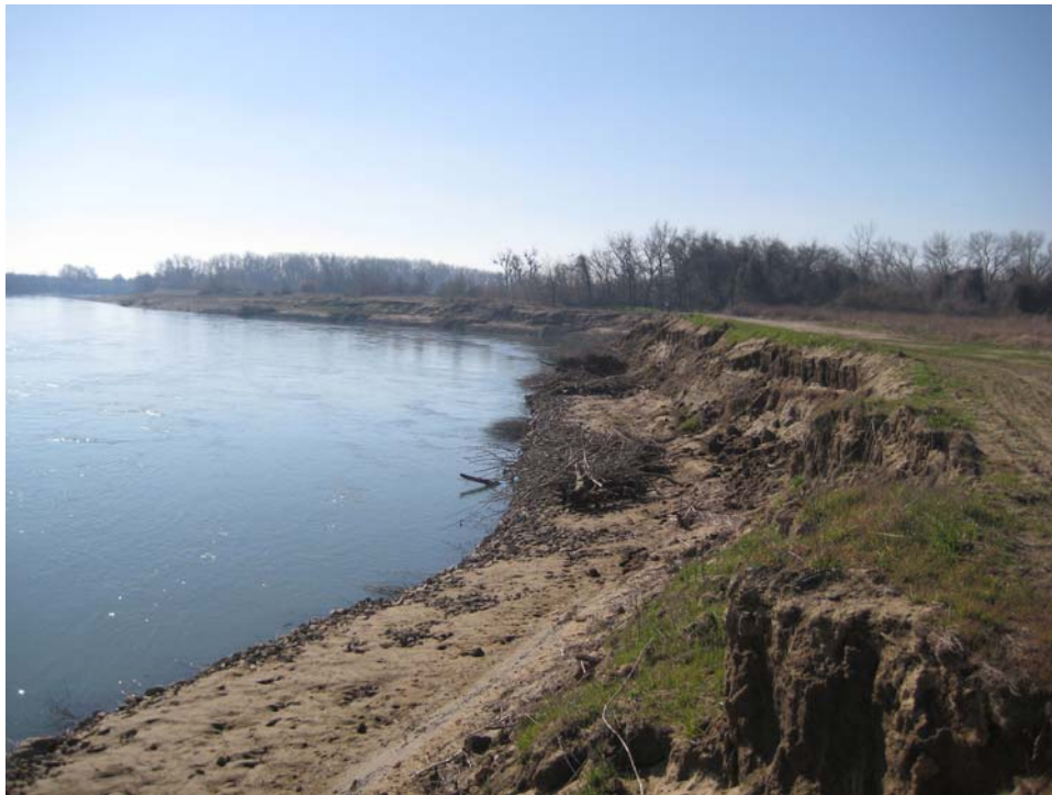
Figure 13. View downstream of bank erosion caused by the first higher winter flows after construction (Photo taken on 03/12/2008).
