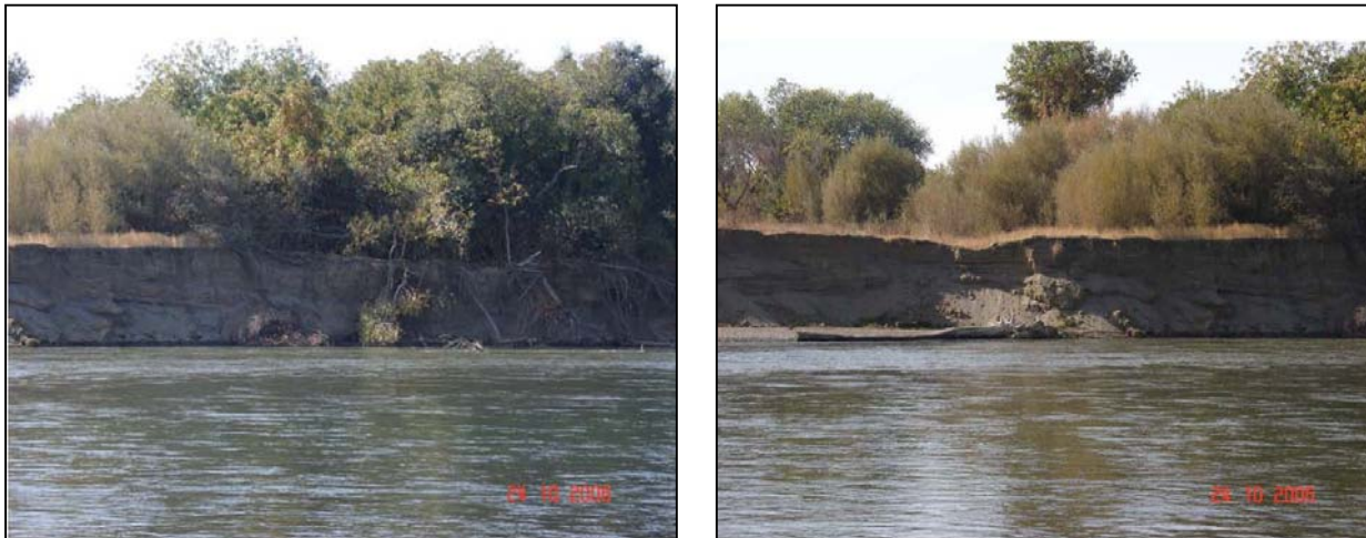
Figure 3.7-5 Photographs of the Apex of the Eroding Bend and the Middle Portion of the Downstream End of the Eroding Bank, Respectively, Prior to Construction of the Rock-toe and Tree Revetment (Photo taken on 10/24/2006) (Tetra Tech 2012a).
