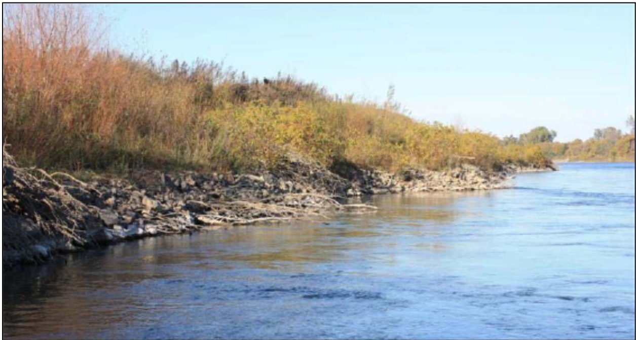
Figure 3.3-3. Upstream View of the Middle Section of the Rock-toe and Tree Revetment, Showing Very Dense Volunteered Riparian Vegetation Species Growing on the Top of the Rock, and the Presence of the Emplaced Large Woody Material on the Top of the Rock and Within the Rock (Source: Tetra Tech 2012a).
