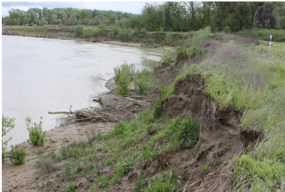
Figure 21. View downstream showing eroding upper bank but no evidence of any scour of the backfill material at the base of the bank. Flow in the river was about 11,000 cfs (Photo taken on 04/12/2008).
