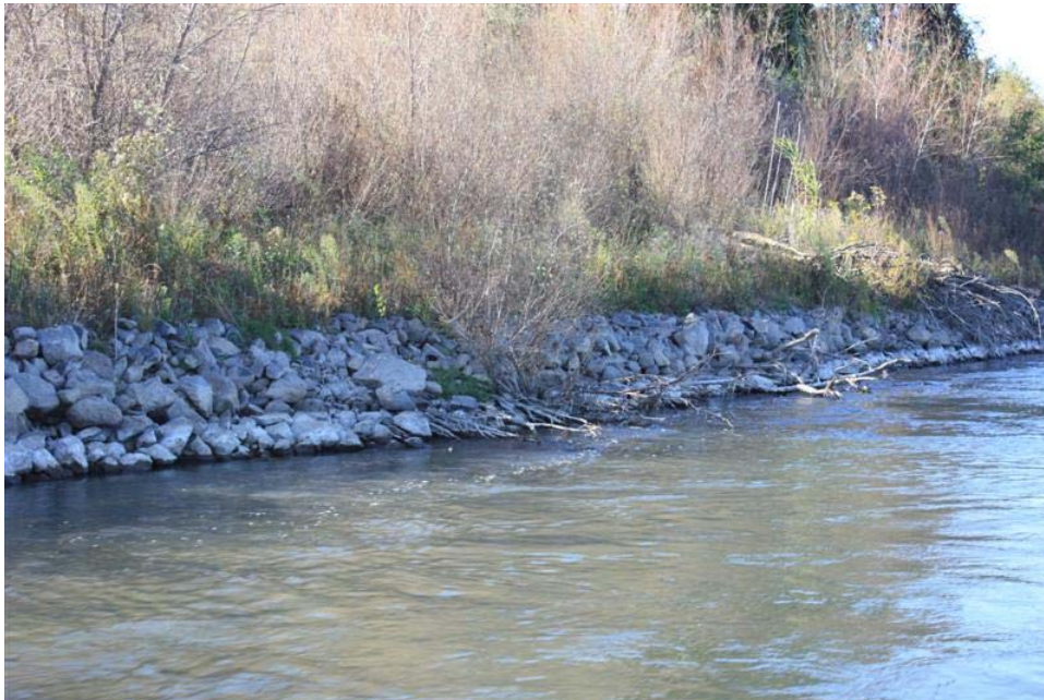
Figure 29. Close up view of the rock toe within the lower end of the revetment. There is no evidence of loss of rock.
