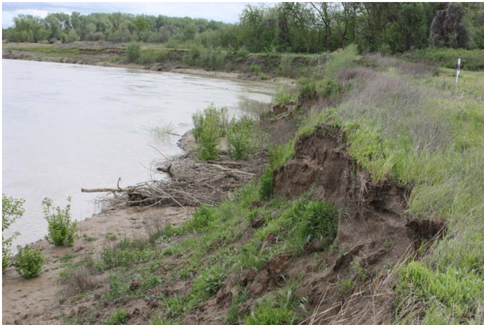
Figure 21. View downstream showing eroding upper bank but no evidence of any scour of the backfill material at the base of the bank. Flow in the river was about 11,000 cfs (Photo taken on 04/12/2010).
