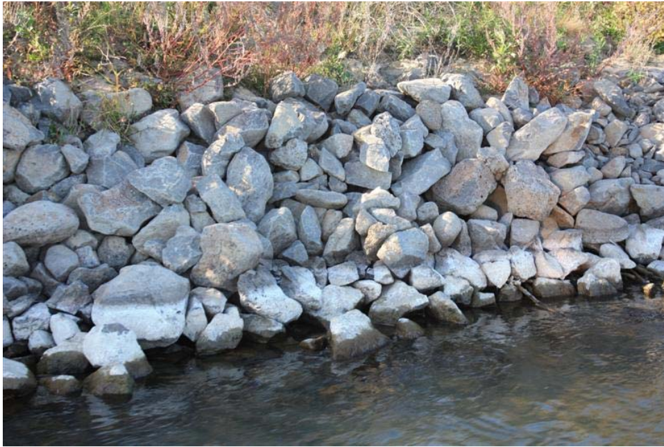
Figure 28. Close up view of the rock toe within the middle section of the revetment. There is no evidence of loss of rock.
