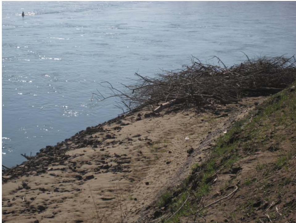
Figure 12. View of intact woody debris on top of the revetment as well as sediment deposition on top of the rock following the first higher winter flows after construction (Photo taken on 03/12/2008).
