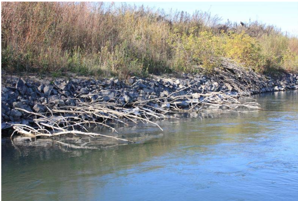
Figure 31. Upstream view of the middle section of the toe rock revetment. Note the large woody debris emplaced on the top of the rock and within the rock during construction.
