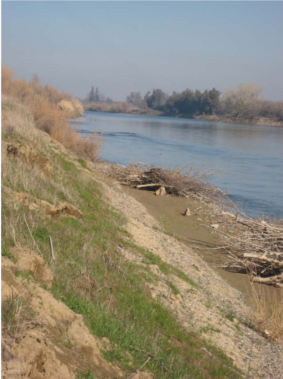
Figure 11. View upstream of the upstream end of the revetment showing the presence of the pre-construction vegetation on the upstream bank (Photo taken on 03/12/2008).
