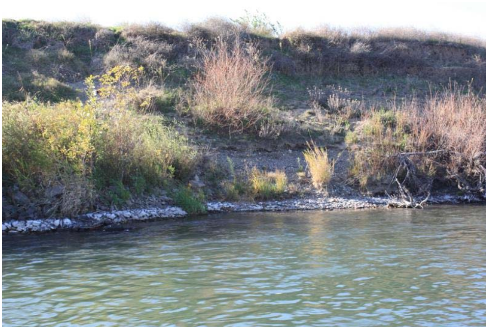
Figure 25. View of the upstream end of the rock revetment and transition to unprotected bank. Note the presence of the willows growing on the bank indicating that there has been little or no erosion at the upstream end of the revetment.
