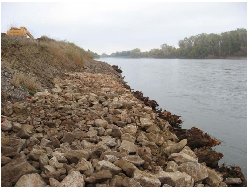
Figure 8. View upstream of the rock toe being emplaced during construction of the revetment. Note the woody material incorporated into the revetment at about Elevation 117 feet (Photo taken on 10/30/2007).
