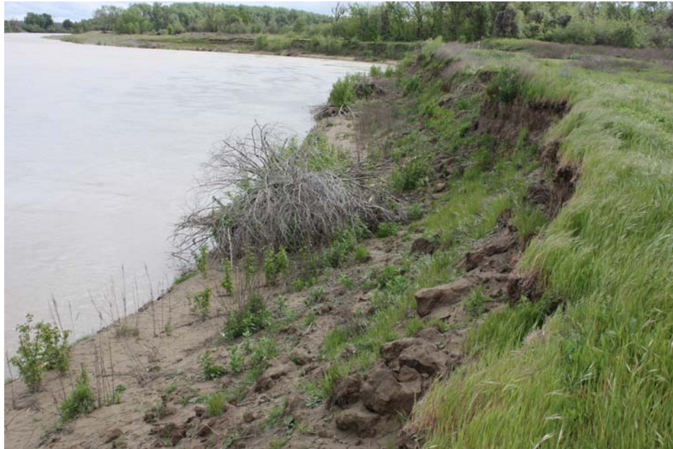
Figure 20. View downstream of eroding upper bank above the top of the revetment that is causing the bank angle to be reduced. Flow in the river was about 11,000 cfs (Photo taken on 04/12/2010).
