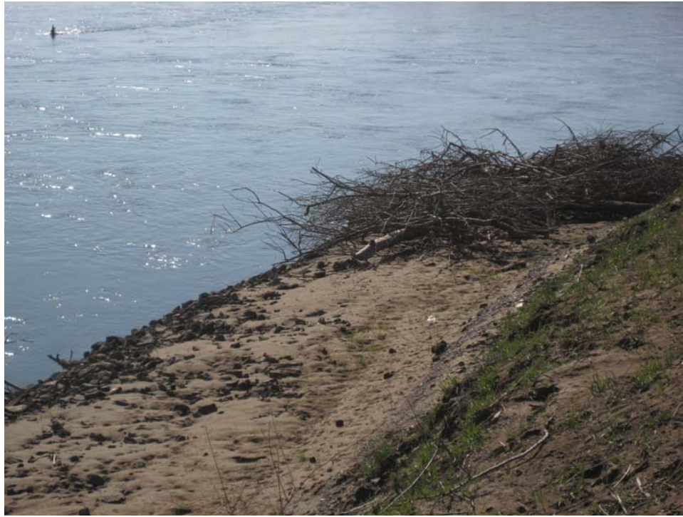
Figure 12. View of intact woody debris on top of the revetment as well as sediment deposition on top of the rock following the first higher winter flows after construction (Photo taken on 03/12/2008).
