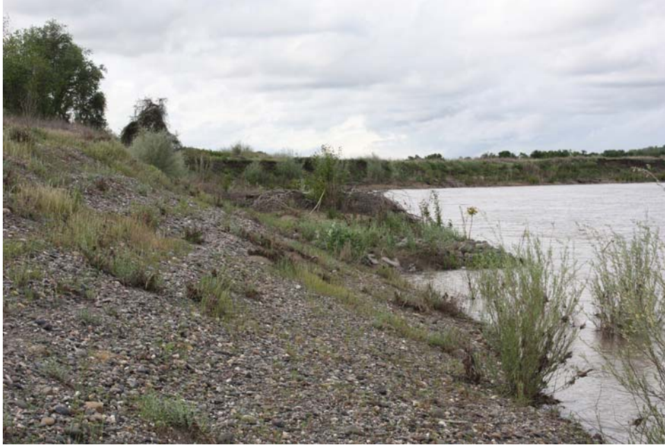
Figure 24. View upstream of the downstream end of the revetment and the downstream tie back. Flow in the river was about 11,000 cfs (Photo taken on 04/12/2010).
