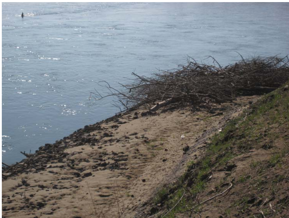
Figure 12. View of intact woody debris on top of the revetment as well as sediment deposition on top of the rock following the first higher winter flows after construction (Photo taken on 03/12/2008).
