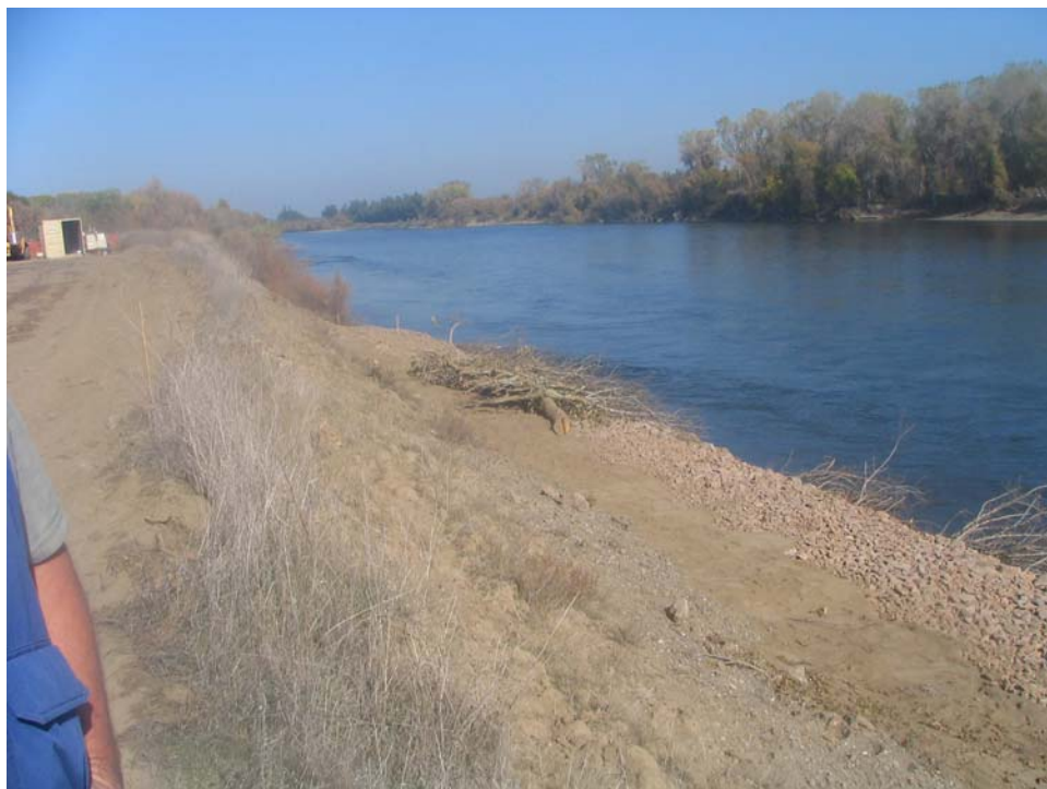
Figure 10. View upstream of backfill in place between the rock revetment and the bank slope during construction (Photo taken 10/30/2007).
