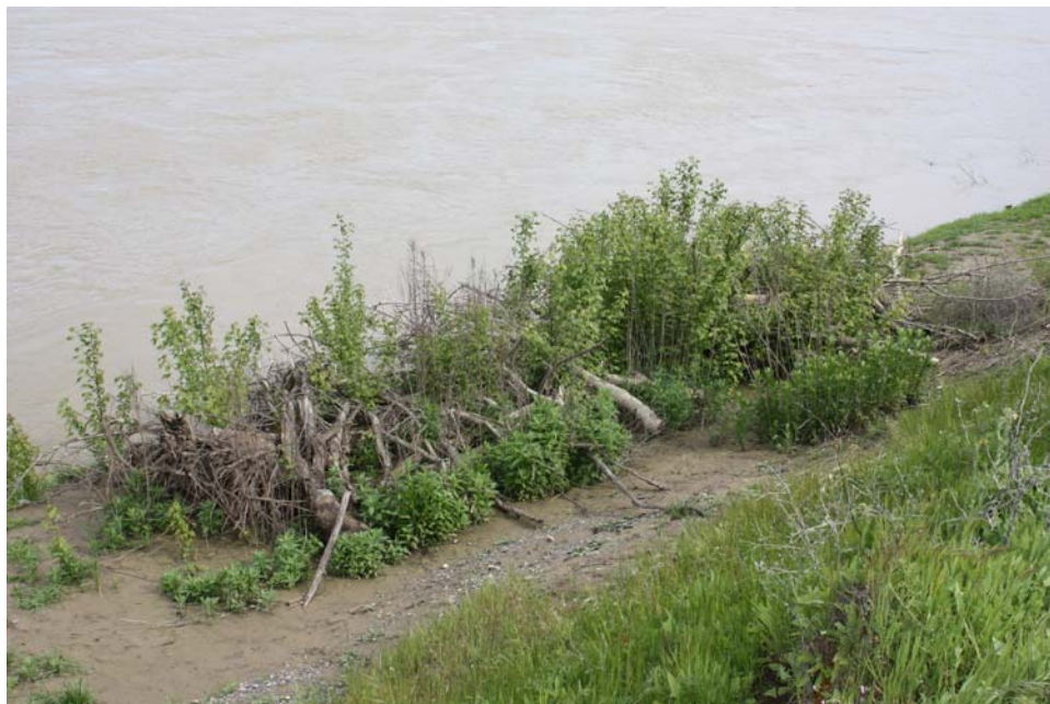
Figure 19. Close up view of a woody debris pile cabled onto the top of the revetment showing volunteer woody plants growing within and around the debris pile. Flow in the river was about 11,000 cfs (Photo taken on 04/12/2010).
