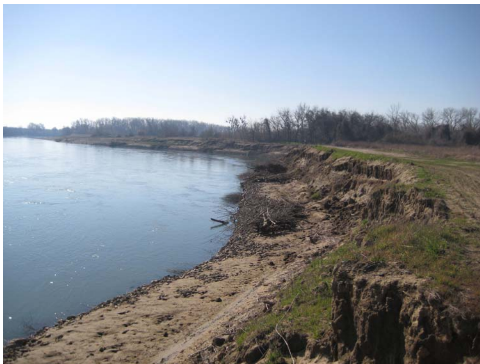
Figure 13. View downstream of bank erosion caused by the first higher winter flows after construction (Photo taken on 03/12/2008).
