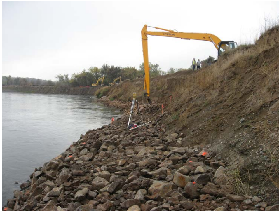
Figure 7. View downstream of the rock toe being emplaced during construction of the revetment. The top of the rock is at Elevation 119 feet (Photo taken on 10/30/2007).
