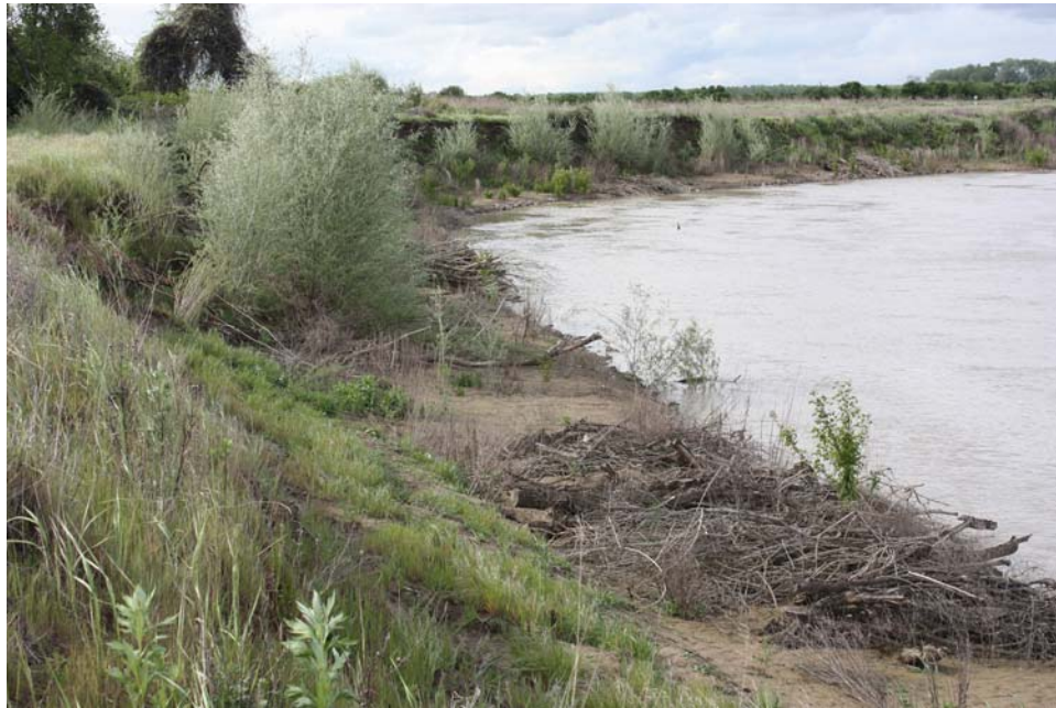
Figure 22. View upstream of willow growth along the top of the revetment and at the base of the eroding bank. Flow in the river was about 11,000 cfs (Photo taken on 04/12/2010).
