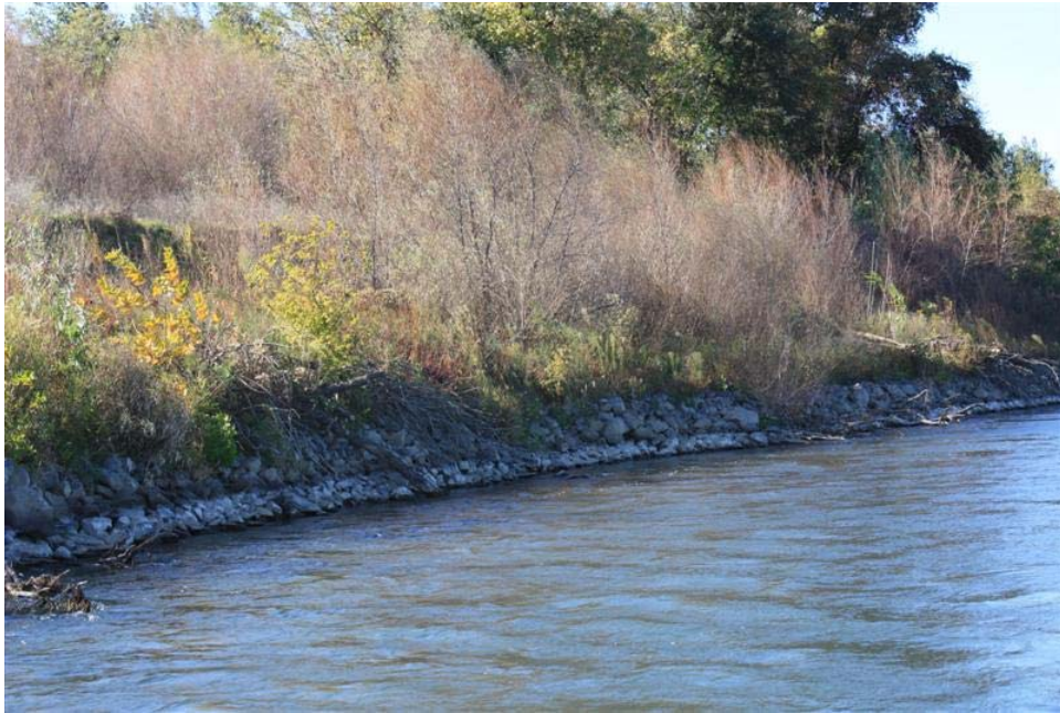
Figure 34. Upstream view of the lower end of the toe rock revetment. Note presence of volunteered riparian vegetation species as well as emplaced large woody debris on the top of the rock and within the rock. There is no evidence of loss of rock from the revetment.
