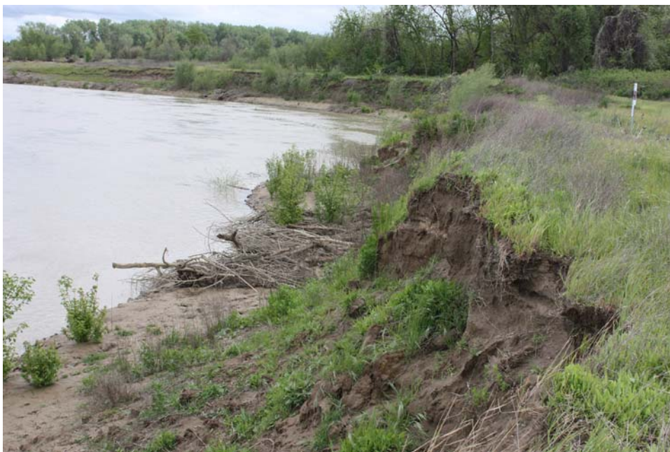
Figure 21. View downstream showing eroding upper bank but no evidence of any scour of the backfill material at the base of the bank. Flow in the river was about 11,000 cfs (Photo taken on 04/12/2010).
