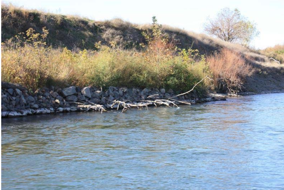
Figure 26. Upstream view of the upstream end of the toe rock revetment. Note presence of riparian vegetation as well as the large woody debris emplaced within the rock during construction. There is no evidence of loss of rock. Note the larger anchor boulders that were used to secure the large woody debris emplaced on the top of the revetment.
