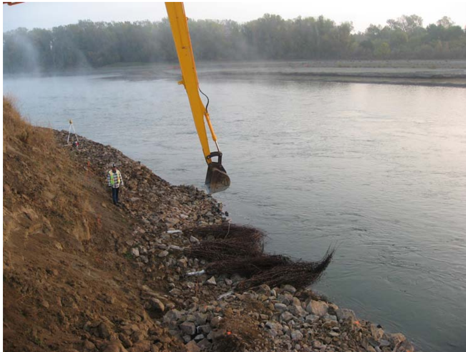
Figure 9. View of woody material being placed on the top of the revetment at about Elevation 119 feet during construction of the revetment (Photo taken on 10/30/2007).
