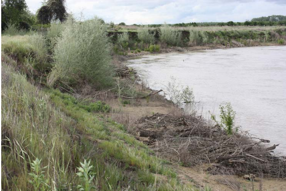
Figure 22. View upstream of willow growth along the top of the revetment and at the base of the eroding bank. Flow in the river was about 11,000 cfs (Photo taken on 04/12/2010).
