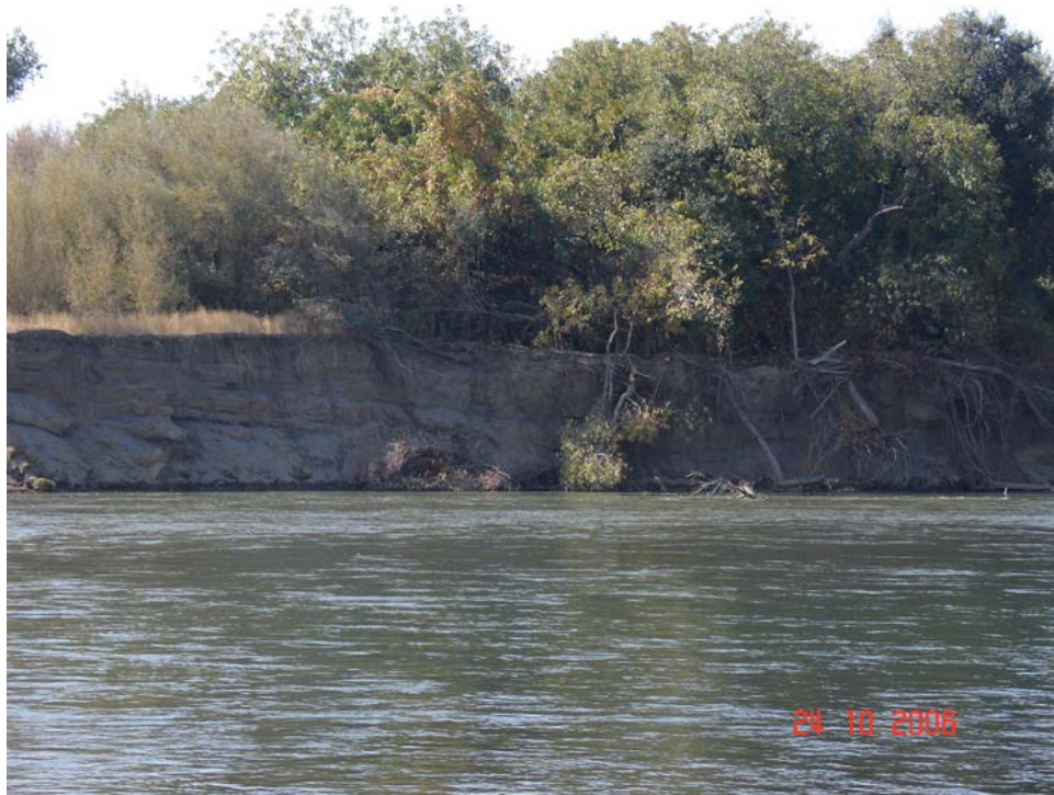
Figure 3. Photograph of the apex of the eroding bend prior to construction of the rock-toe/brush revetment (Photo taken on 10/24/2006).
