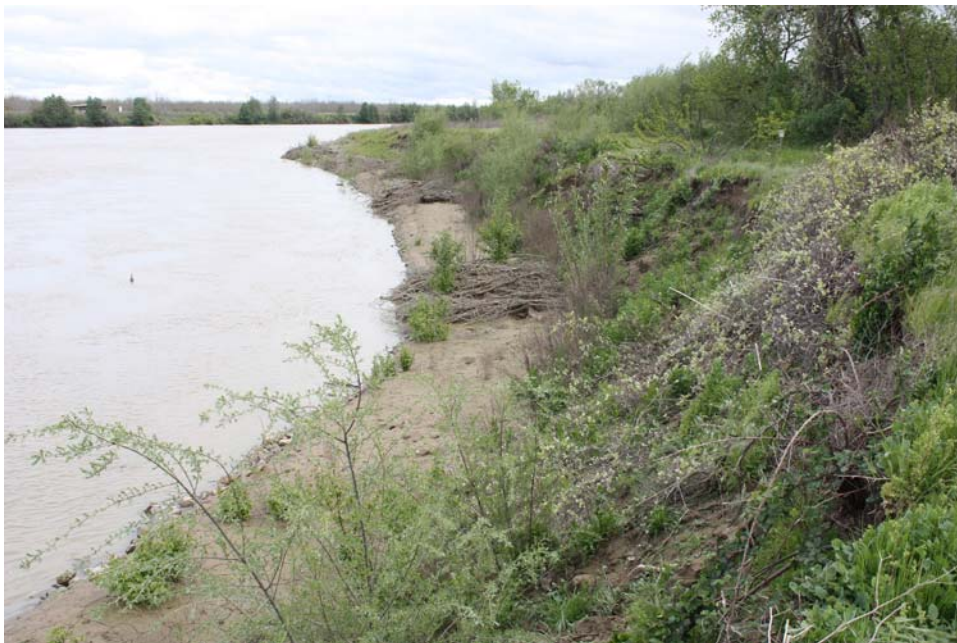
Figure 23. View downstream of the downstream part of the revetment with vegetation growing at the toe of the bank and on the top of the revetment. Flow in the river was about 11,000 cfs (Photo taken on 04/12/2010).
