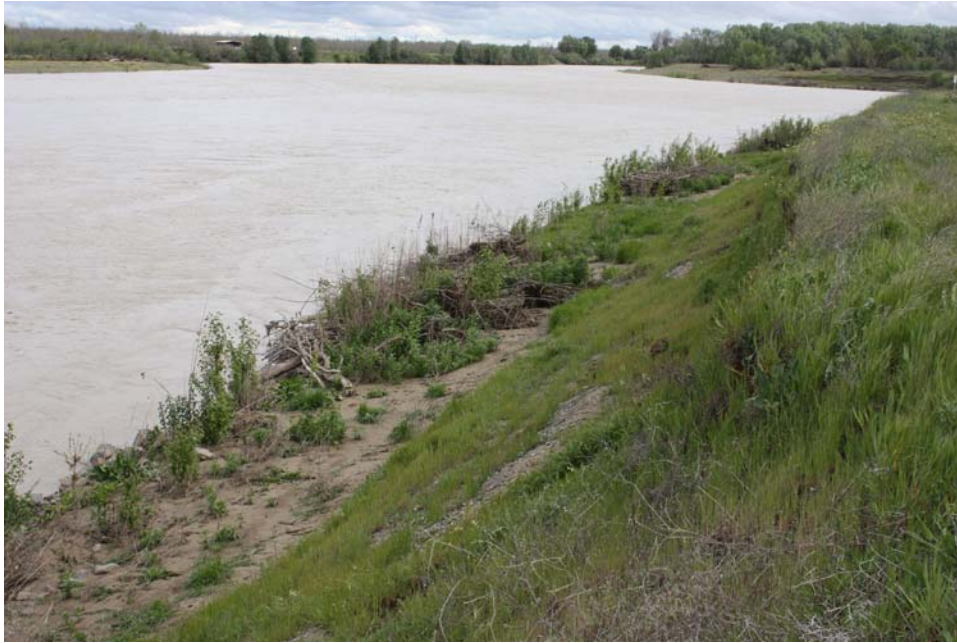
Figure 18. View downstream of the top of the revetment showing the woody debris piles that were placed and cabled onto the revetment. Flow in the river was about 11,000 cfs (Photo taken on 04/12/2010).
