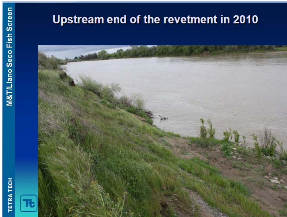
This slide shows there is no flanking at the upstream end of the revetment.
