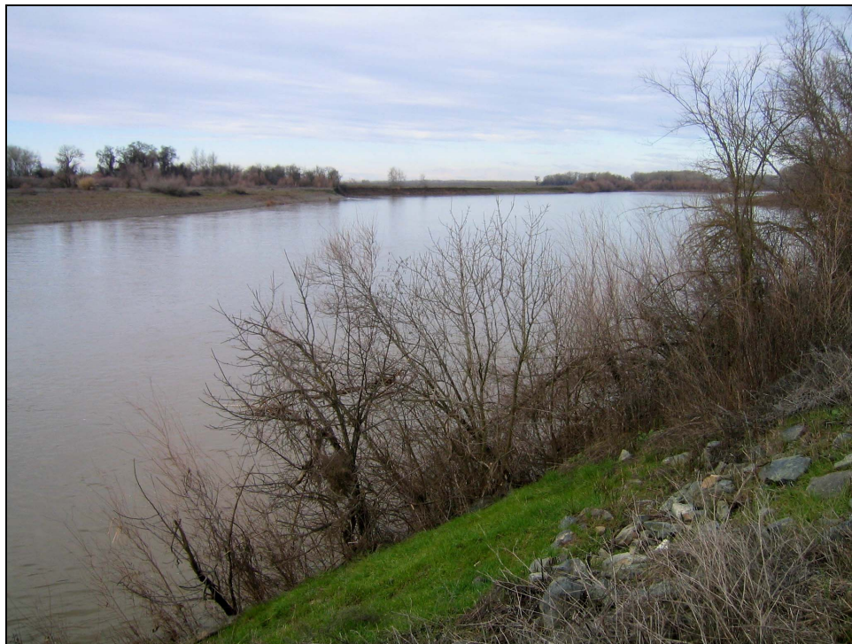
Figure 3. View looking upstream toward the eroding right bank of the Sacramento River at RM 192.8 across from the location of the M&T intake and Big Chico Creek.
